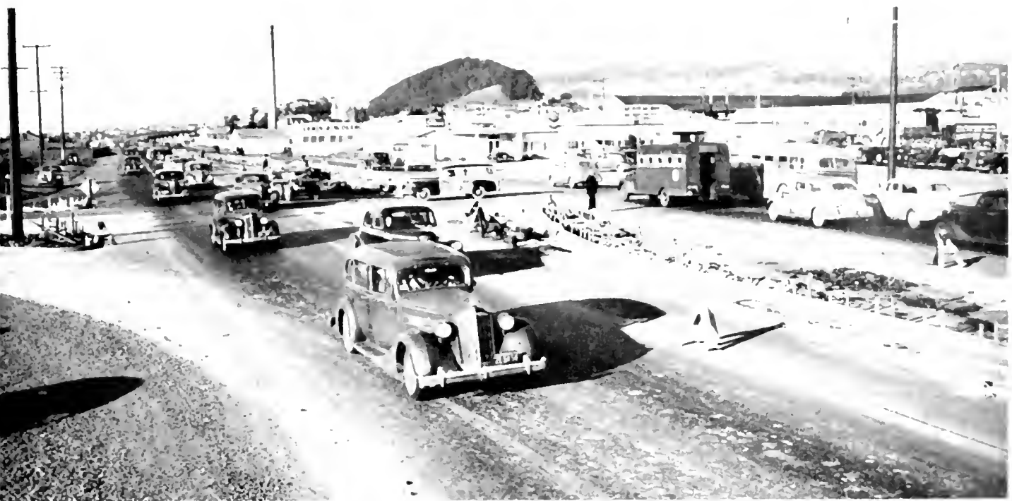
Intersection of East Shore Highway and Gilman Street, showing island in process of construction. Automatic signals will be installed at this point
